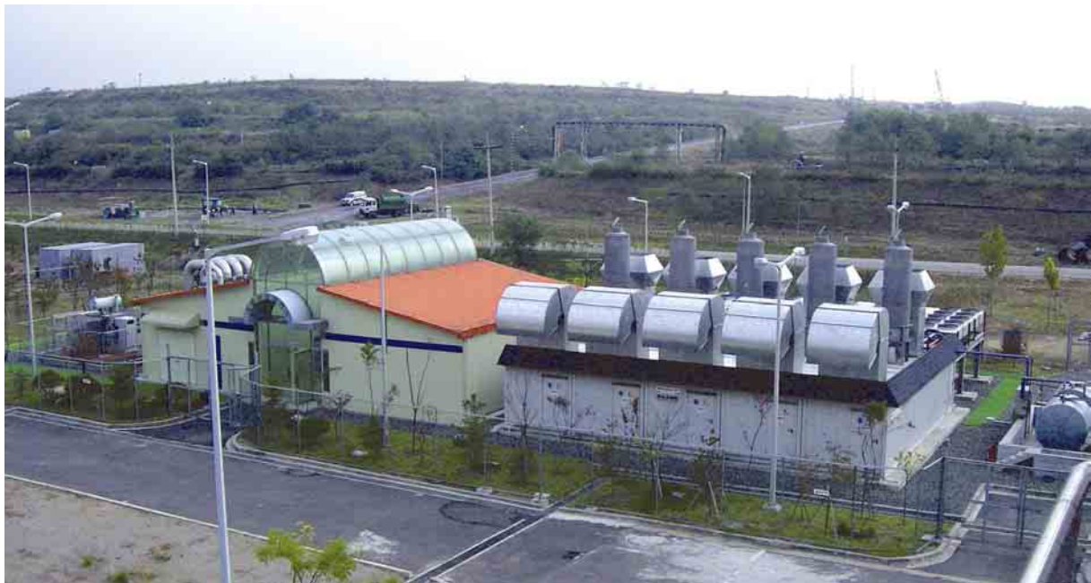
Fig. 9: First stage of construction with 5 CHP modules. Operation building on the left hand side.
