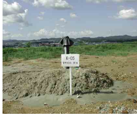
Fig. 5: New vertical gas well
