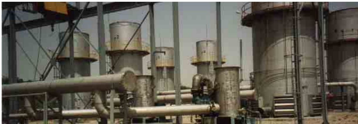
Fig. 3: Old flare unit installed on the Sudokwon landfill site, Seoul (Korea)
