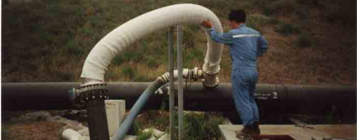
Fig. 7: Horizontal gas well connected to the circular pipeline: old gas extraction system.
