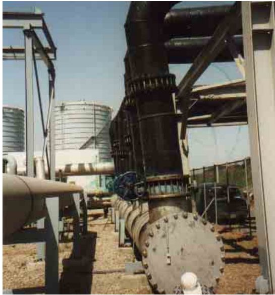
Fig. 4: Old manifold for circular pipelines
