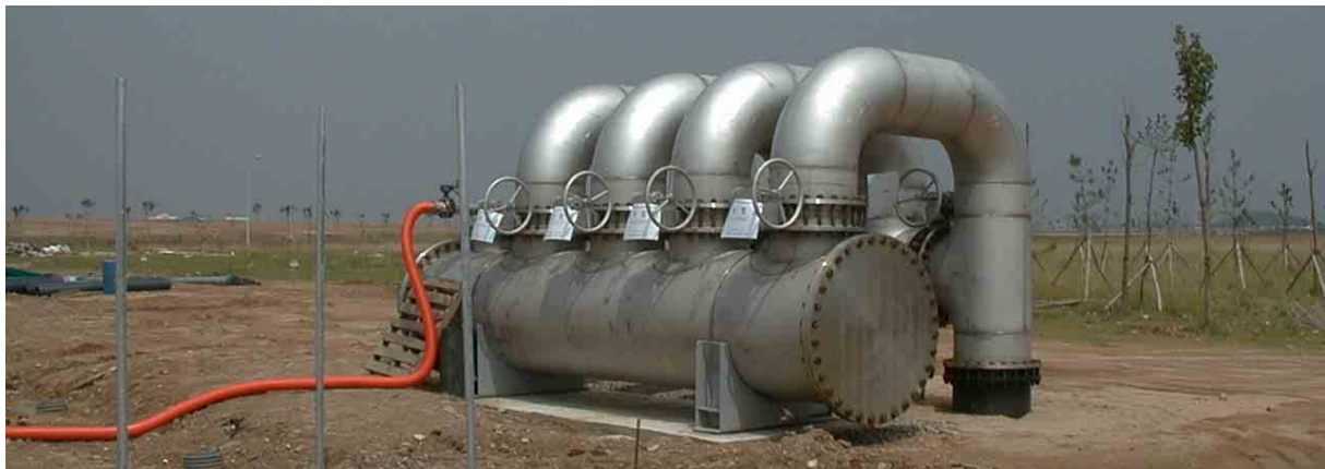
Fig. 8: Gas manifold joining circular pipelines from Area 1 and 2
