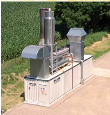
above: The HAASE „Energy Center“ container unit also encloses gas cooler, analysis, booster, flare, and the CHP control system.
