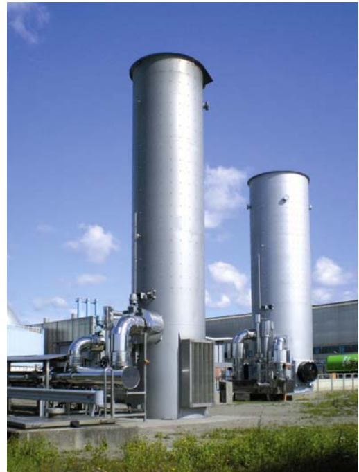
Picture 2: HAASE sludge gas flares Next to the flare operating since 2004 (left, 17MW), an additional flare was installed (right, 27MW). It is furnished with a two-stage burner and a pilot burner for midjet quantities
