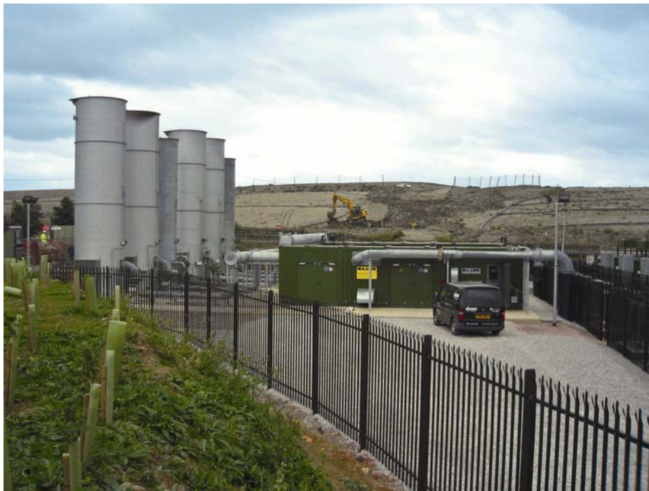
Picture 3: 6 landfill gas flares on Brogorough landfill site, England Total combustion capacity 60MW. The appending gas booster station supplies 13,800m 3 /h of landfill gas
